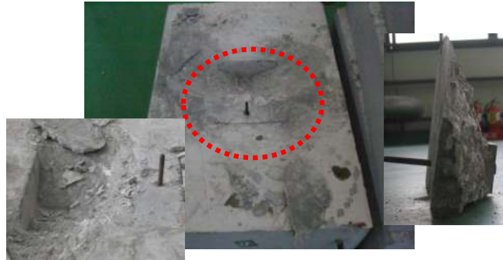
Concrete cone failure (crack model)
