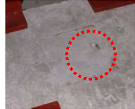
Tensile failure of bolt (no crack model)
